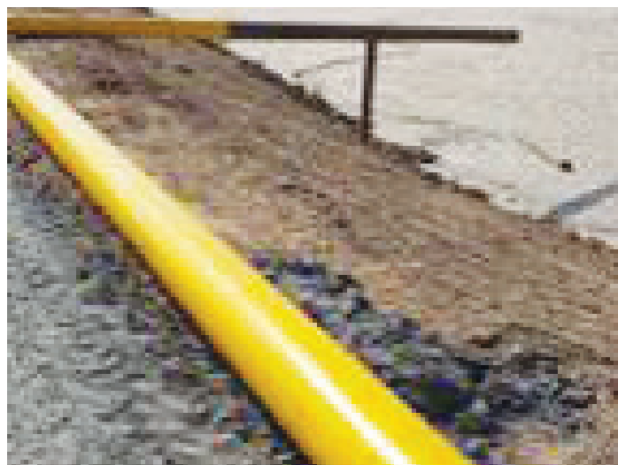
Fig. 4: Rampura-Agucha and Rajpura-Dariba Pb-Zn Mines Tailings Facilities (with about 50% solids) from the beneficiation plant are disposed in environmentally safe manner in tailing dam. Tailing dam stability study carried out by experts. Impervious layer on bottom & sides of the dam is provided to eliminate the possibility of any seepage. Regular groundwater monitoring and concurrent recycling of water is done for plant use. [Photo source: Sudesh K. Wadhawan]
