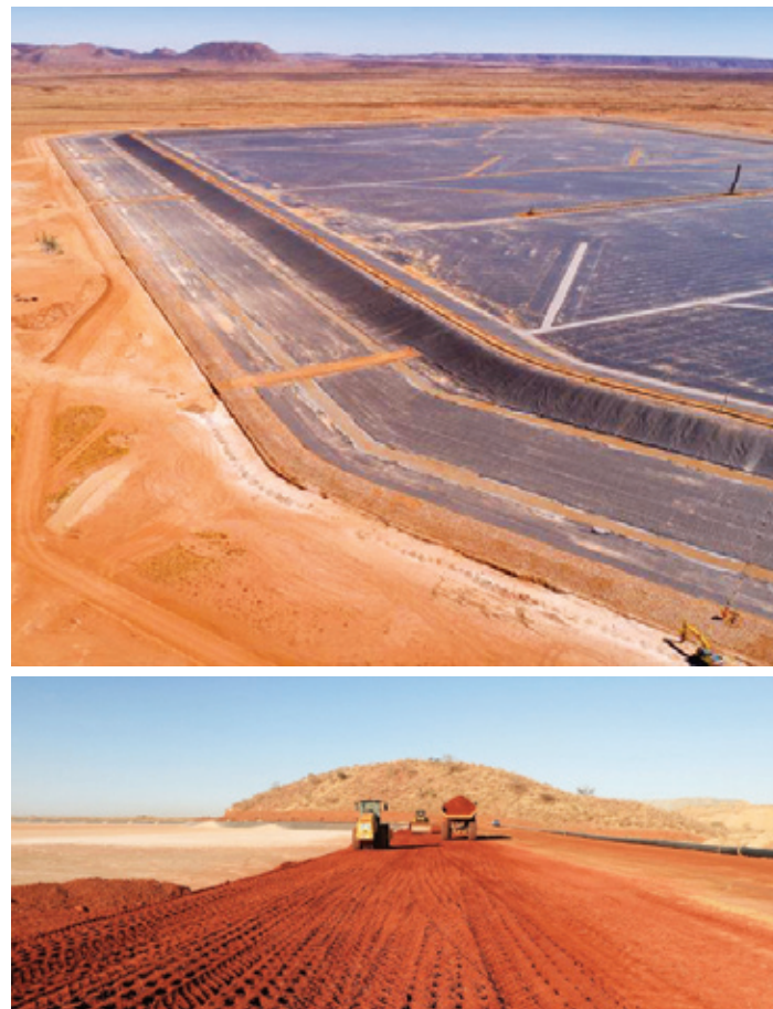
Fig. 3: Vedanta Gamsberg TMF - Gamsberg Zinc Mining and Concentrator Project located in Aggeneys, South Africa [Photo source: Wikipedia, Vedanta Report, 2019]
