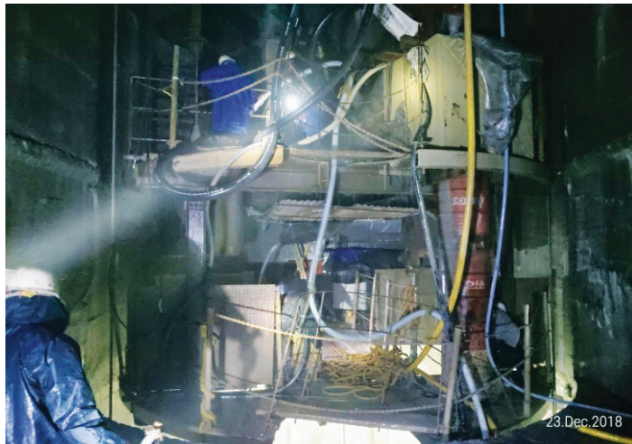
Fig. 3: Pumping arrangement (underground) at SVS site
