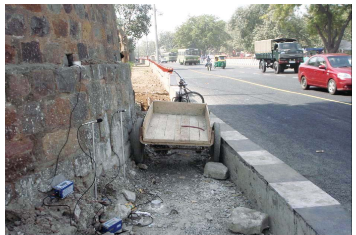
Figure 9. Installation of seismographs for measurement of road traffic induced vibration (Source: CIMFR Report No. CNP/R/2862/2011-12)
